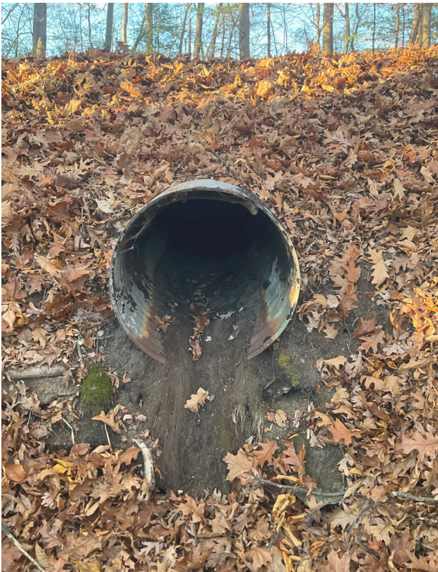
Fg 12. Culvert CU061 - Section Loss
