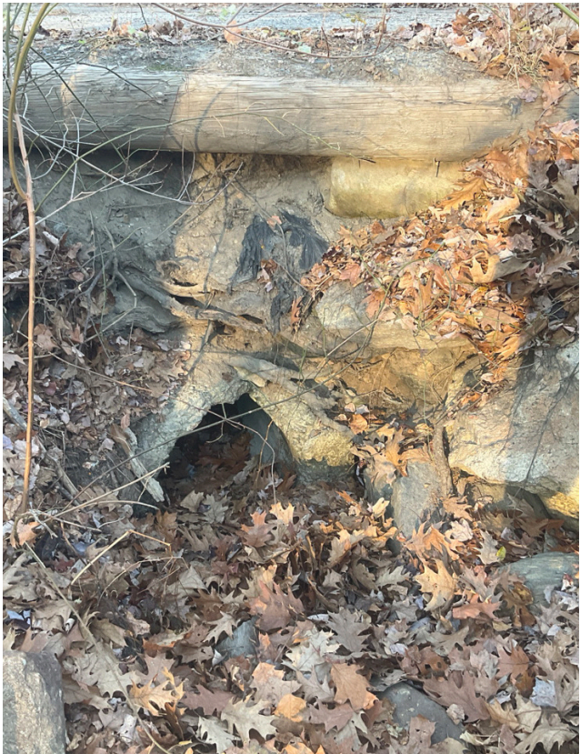
Fg 11. Culvert CU073 - Spalling Pipe
