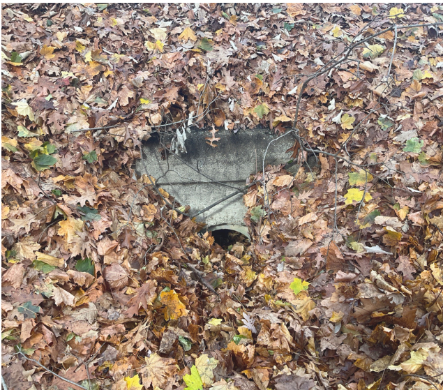
Fg 6. Culvert CU135 - Inlet 75% Obstructed
