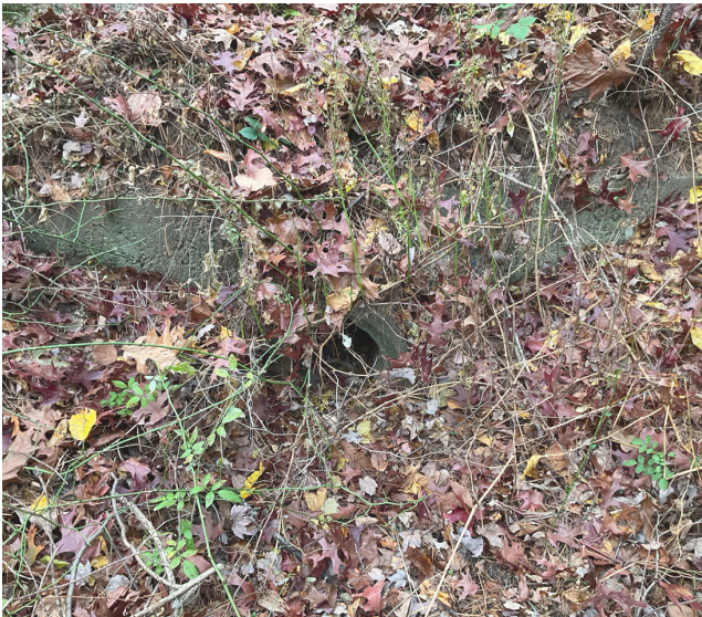
Fg 8. Culvert CU050 - Vegetation Overgrowth
