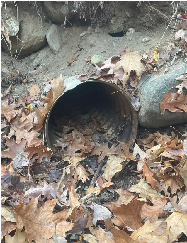
Fg 13. Culvert CU047 - Missing Headwall Stones
