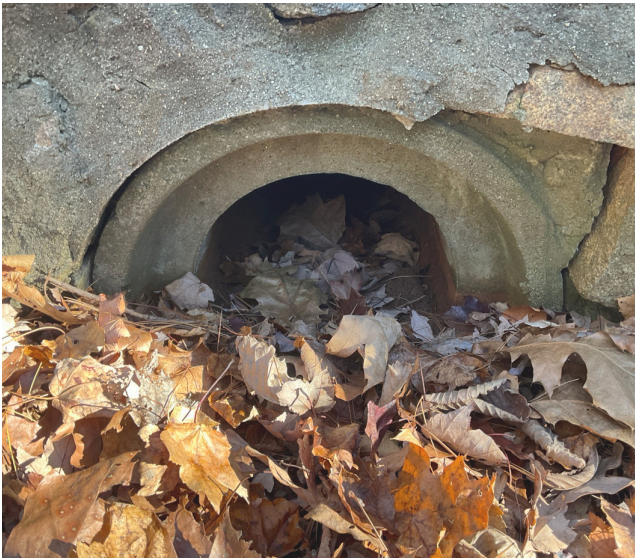
Fg 4. Culvert CU109 - Outlet 20% Obstructed
