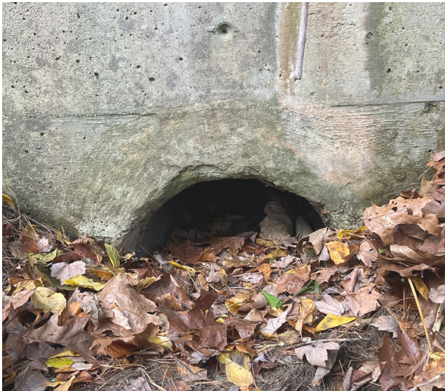
Fg 5. Culvert CU036 - Outlet 50% Obstructed
