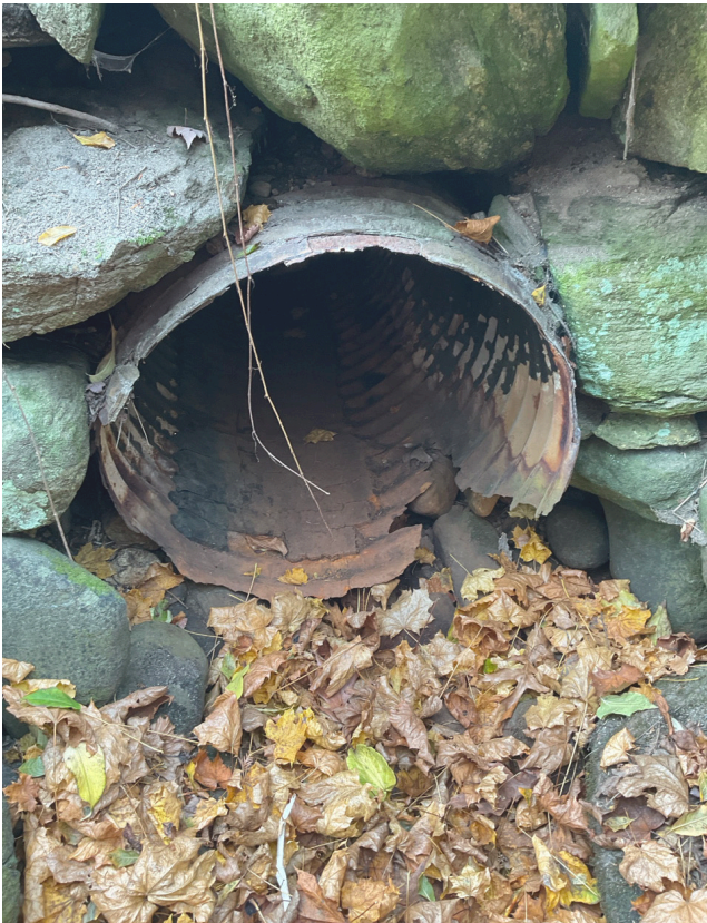
Fg 10. Culvert CU015 - Rust and Section Loss
