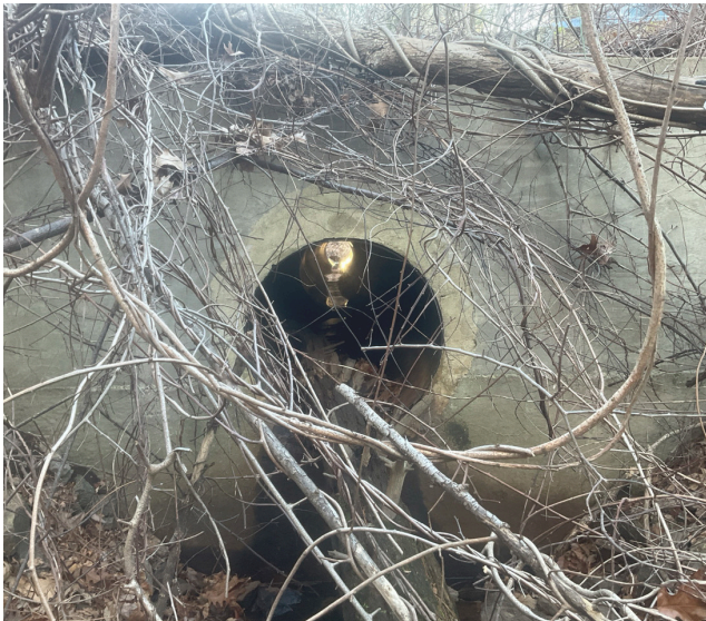
Fg 9. Culvert CU154 - Outlet Blocked by Branches
